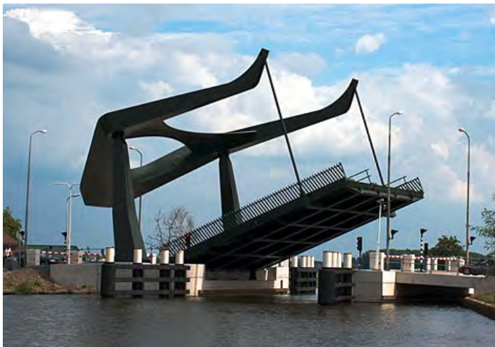
OPENING BRIDGE „PRAYER OF SHADOW“: The spectacular bridge over the Amstel is coated in RAL 6007 Bottle green. Within the space of a minute, this high-tech-bridge in Vrouwenakker (south of Amsterdam) can be raised or lowered.
